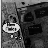
Construction began on a new athletic field complex to be located across the street from the university's Sassafras housing units. The project will include a softball field, a synthetic surface multipurpose field equipped with lights, and a grass-surface multipurpose practice field. The fields are expected to be ready for use in the 2004-05 academic year.
